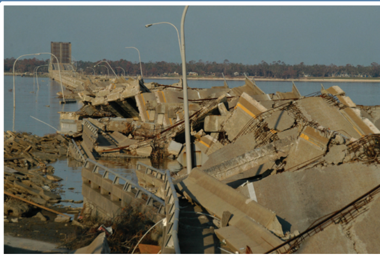
Biloxi, Mississippi, November 3, 2005 – The Hwy 90 bridge from Biloxi to Ocean Springs lies in a twisted mass as result of catastrophic wind and storm surge from Hurricane Katrina. Road closure along the coastal area has complicated recovery efforts. FEMA Photo by George Armstrong
